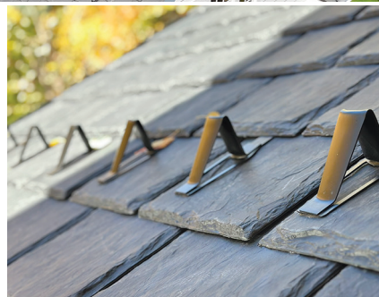
RIGHT: DaVinci Single-Width Slate roof with Everest EG16 snow guards in Dark Bronze placed in a Soldier Row pattern on the roof to help break up snows as they slide and melt off the composite roof.
