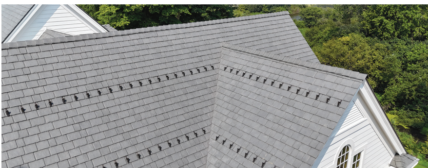
ABOVE: Rocky Mountain Snow Guards installed in a Soldier Row Pattern on roof help provide barriers so that melting snows on roof do not release all at one time.
