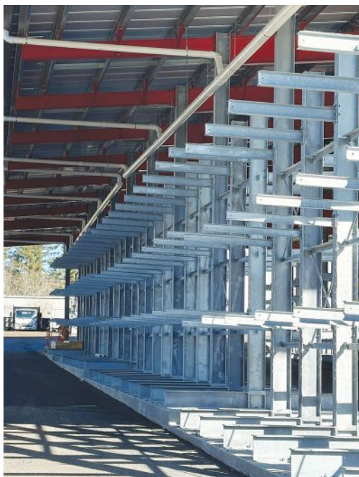
Krauter Auto-Stak reports an uptick in requests for galvanized cantilever racks and rack canopies. It recommends a fresh approach with a high density system that could improve the SKU count and increase labor productivity.
