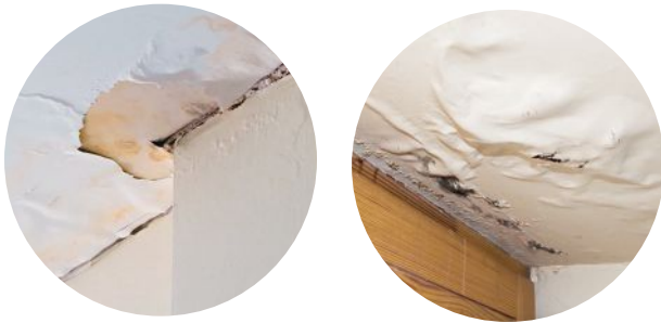
Damage caused by conventional boot failure
