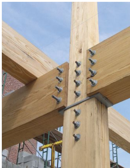
RIGHT: The Power Column from Anthony Forest Products is becoming increasingly popular in mass timber wood framing systems in commercial or multifamily applications.
